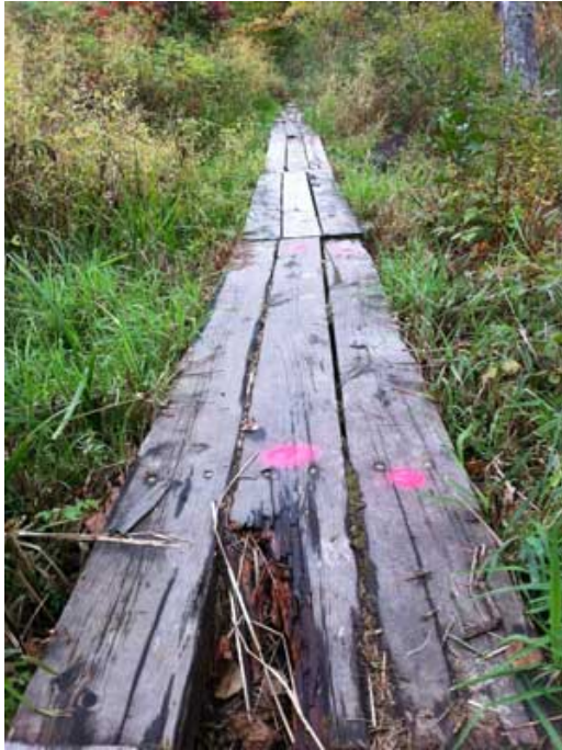
A bridge in need of repair.
